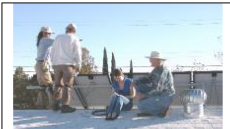
On the roof...Positive Energy, Inc. installers discuss the installation while Bobbie Hutson talks to reporter Bethany Conway of the Las Cruces Bulletin
